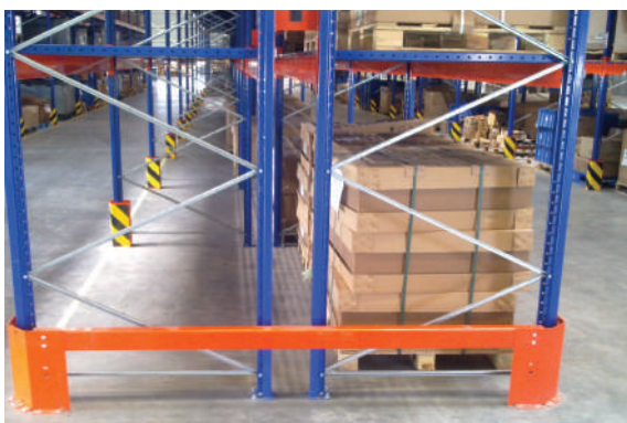
Aisle Raw guards for Frame safety while equipment drive
